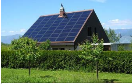
Example of a Solar Conversion System, Structure-mounted
